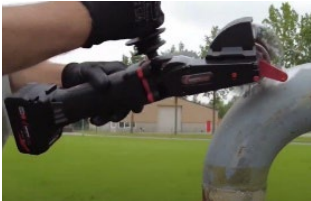
How to Remove Rust and Corrosion at Heights?
